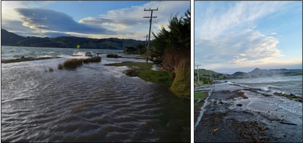
Figure 5 & 6 Tidewater Drive in Harwood is a low-lying where the current sea wall is inadequate to protect people or property from storms, high tides and sea level rise.
